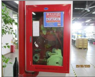
Photo of fire safety equipment 43 Fire hydrant.JPG
