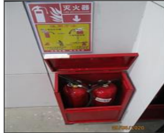
Photo of fire safety equipment 41 Fire extinguisher.JPG
