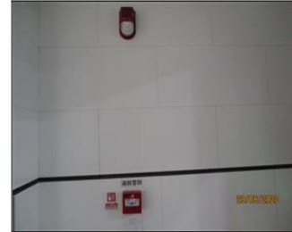
Photo of fire safety equipment 42 Fire alarm bell.JPG
